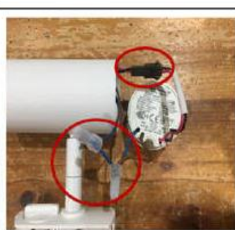
Figure2 Loose the connection
