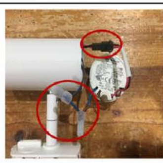
Figure2 Loose the connection
