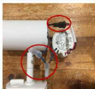
Figure2 Loose the connection
